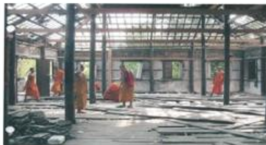
Left. Construction of new school for monks. Lower left. Village children setting up desks. Lower right. First bathrooms ever built in Pagoda Thmey
